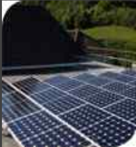
Solar photovoltaic (PV)
