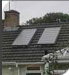
Solar thermal hot water
