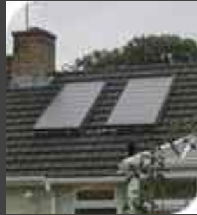
Solar thermal hot water
