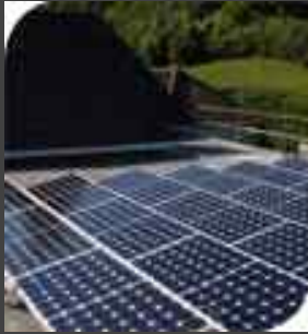
Solar photovoltaic (PV)
